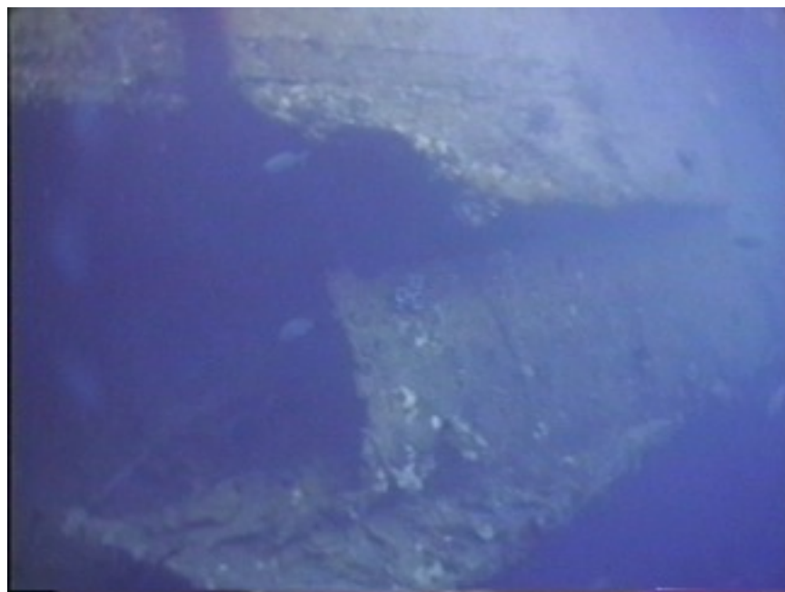
Photo KS13-3 Hole in hull bottom on port side near the end of the bilge keel. Divers can drop straight down through this hole into the shadows of the ship for excellent photos of marine life in open water below.
