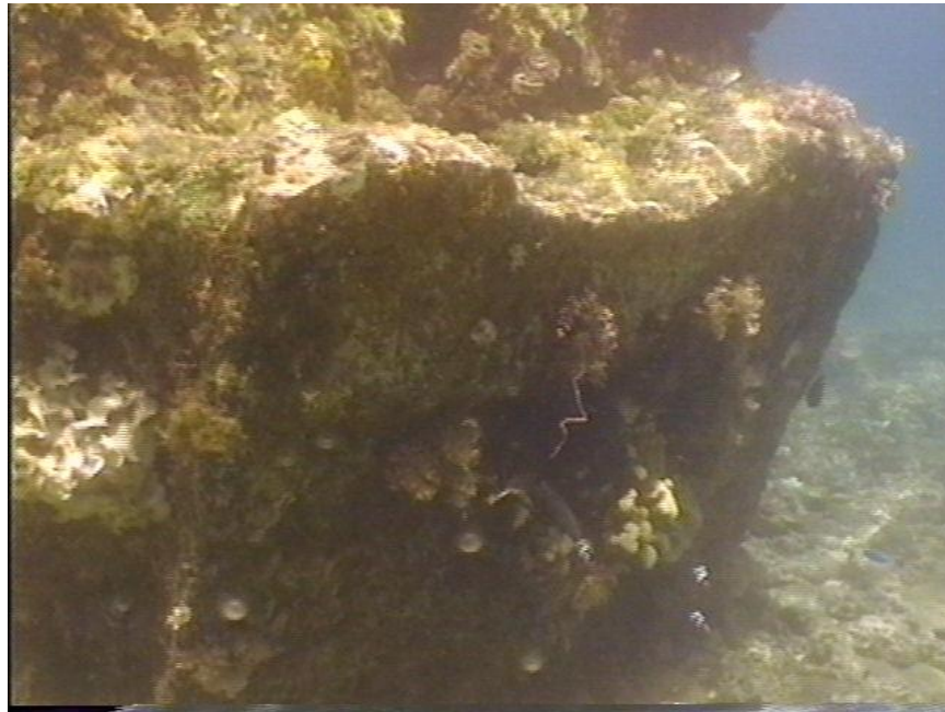
Photo MS4-5 Top of concrete "Dead-man" rolled over into deeper water.
