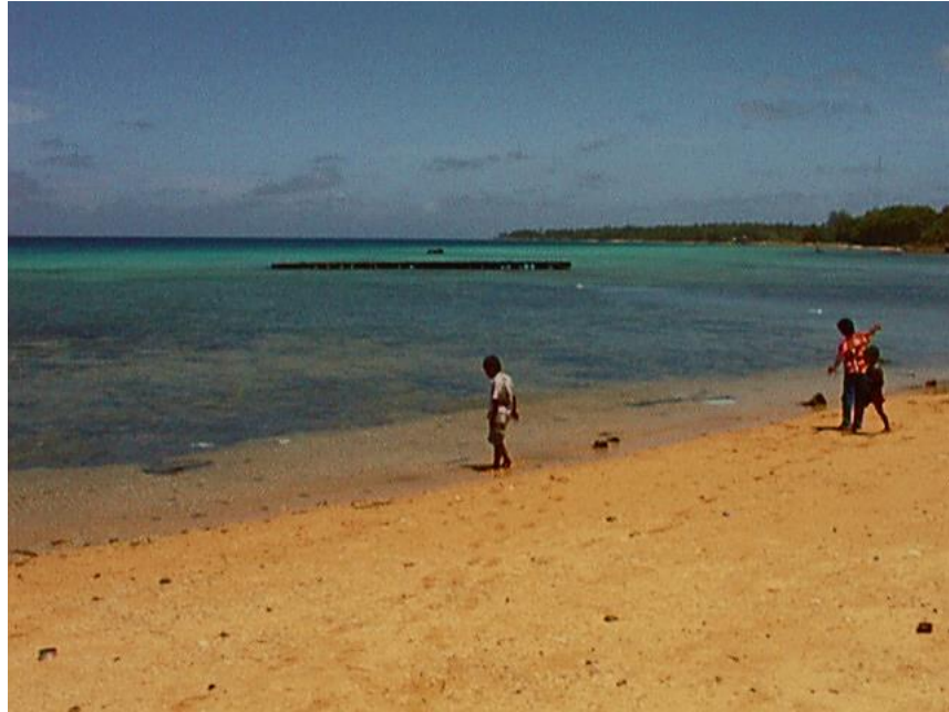
Photo MS6-2 A broken section of Rita US Dock lagoon-side of the shore-side anchoring point The "Dead-man" on the end of the Japanese Wharf is visible farther behind it, and also the Majuro Site 3 "Parking Lot" directly in line with a compass point ( 260 degrees ) to the post on the shallow coral area near
