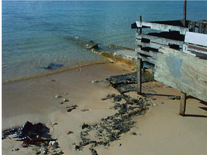
Photo MS8-2 North side of Seaplane Ramp with remains of Marston Matting still embedded in the ground. A pig pen has been secured to the concrete section.
