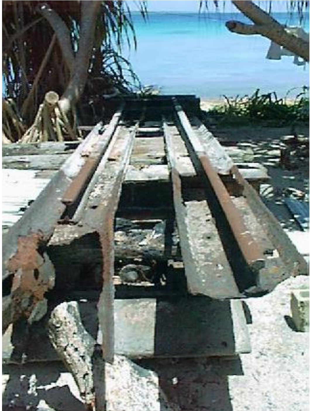
Photo MS7-1 Shore side end of Marine Railway, north track section. Note the sheet pile and heavy timber foundation.
