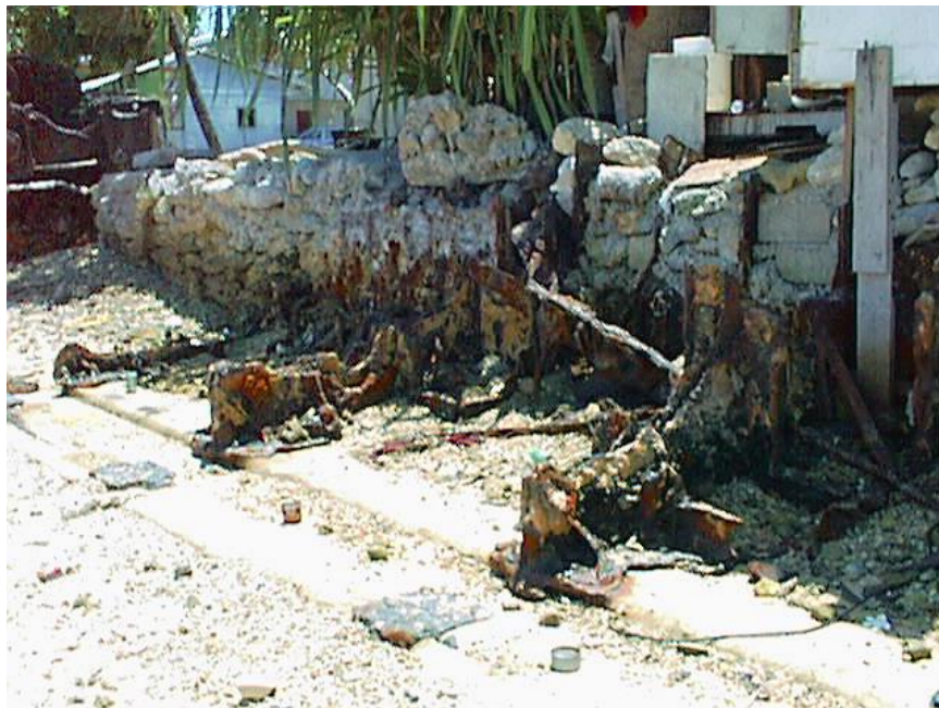
MS6-1 Shore-side attachment point on the US dock at Rita. A section of barge was set in concrete on the hard reef at the shore-line.
