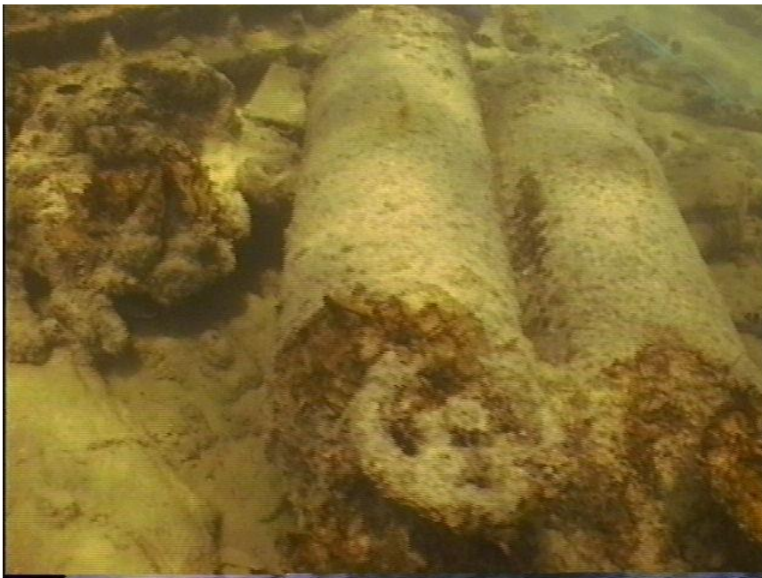
Photo WT11-5. Air tanks to start main engine and/or generators.
