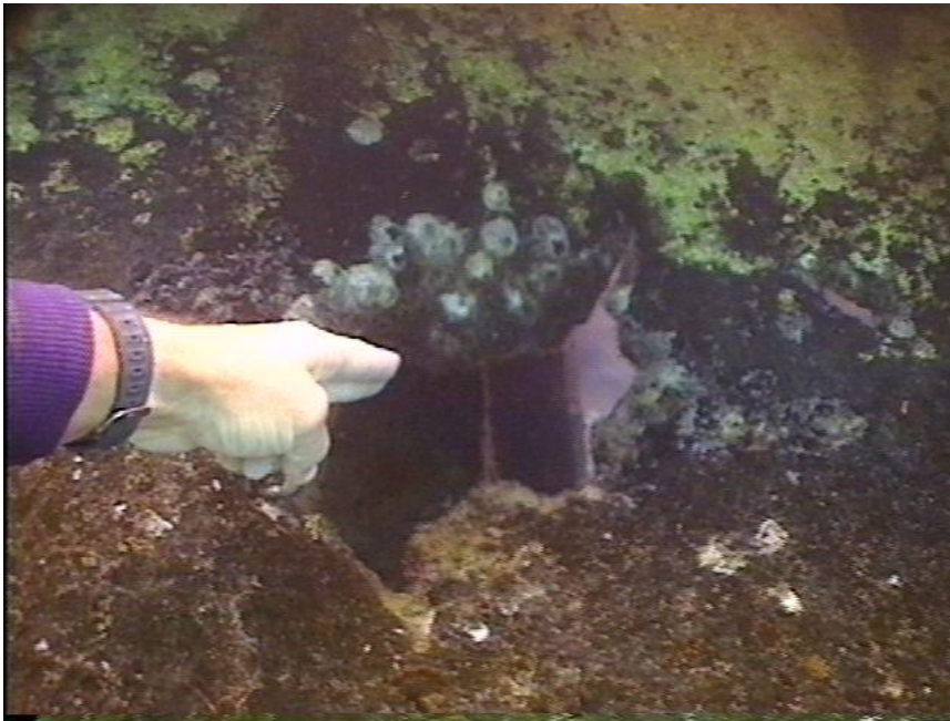
Photo WT13-7. Hole likely from artillery shell, but also possible damage from a near bomb explosion.
