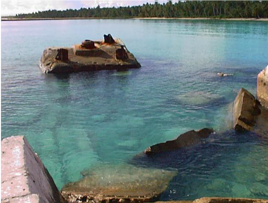
Photo WT6-2. Deep end of Main Service Dock, heavily damaged by bombing and time, with crane base exposed on original end of dock.
